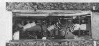
Plenty of room for radio installation.
