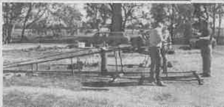
Nagambie tower construction Graeme Sinclair (back to camera) Geoff Lawson far right. Flying field through trees in background.
