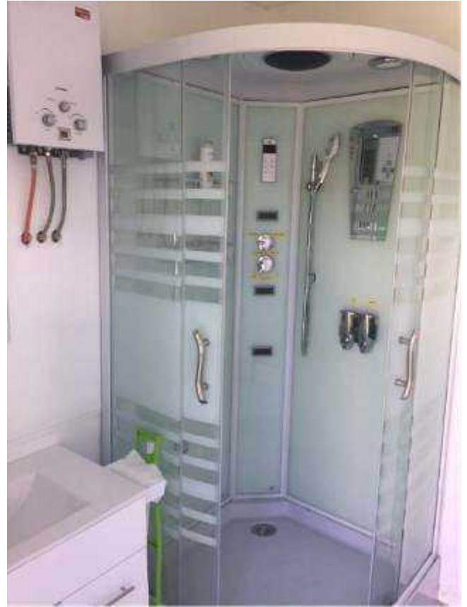
NAAS shower facility.
